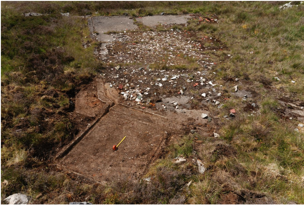
77. Light surface excavation revealed the porch base. Note drainage channels in concrete, which appear to have run on the inside of the building's skin. The drain for the whole building emptied at the lower far left corner of the porch. Porch is 5' wide (outer edges) by 69½" (to outer edge of drain channel). Tape open to 2'.
