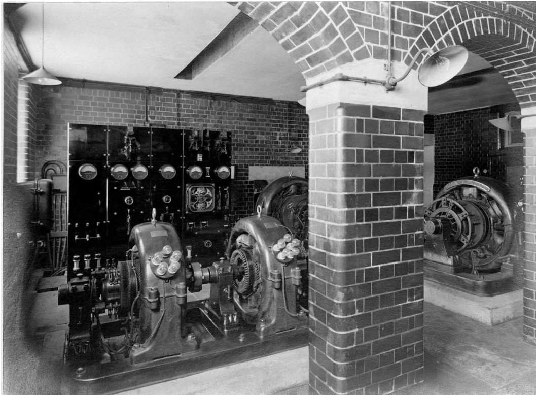
C36. Leeds Firebrick Co bricks in place within the transmitter buildings, providing for a practical, cleanable surface around machinery.
