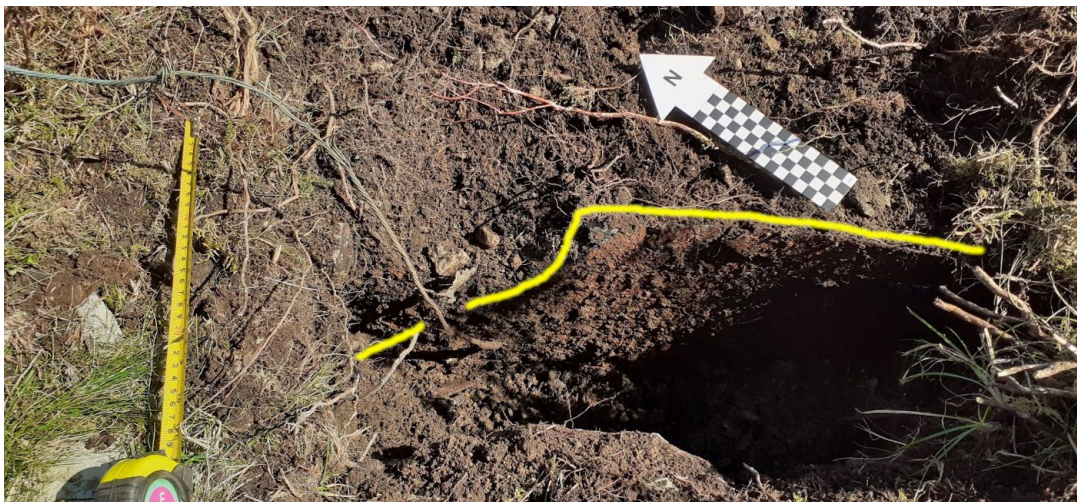
D13 , below: detail of wire connection to plate, the upper plate edge highlighted in yellow line. Tape open to 1ft, north indicator scale in cm squares.
