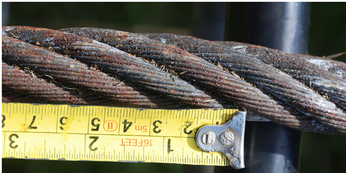
19. 1" diameter stranded stay cable – usually then termed 3" [circumference] cable – was discovered, buried at the western foot of the octagonal concrete base (see 108 ) during fieldwork. for this study.
