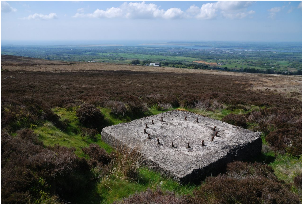
95. Concrete baseplate mounting block (Mast 6), with 16 bolts of 2" diameter at 14.5" centres protruding 4.25" in a ring 6 feet in diameter. 53.123082°, -4.182320°.
