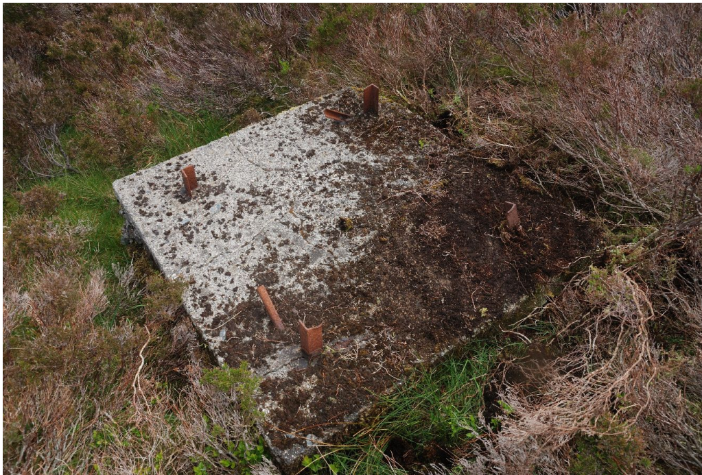
105. A clear example of a 1923 counterpoise lattice mast base, with remnant steelwork. Concrete base of 4'x4', lattice of sides 32" x 32".
