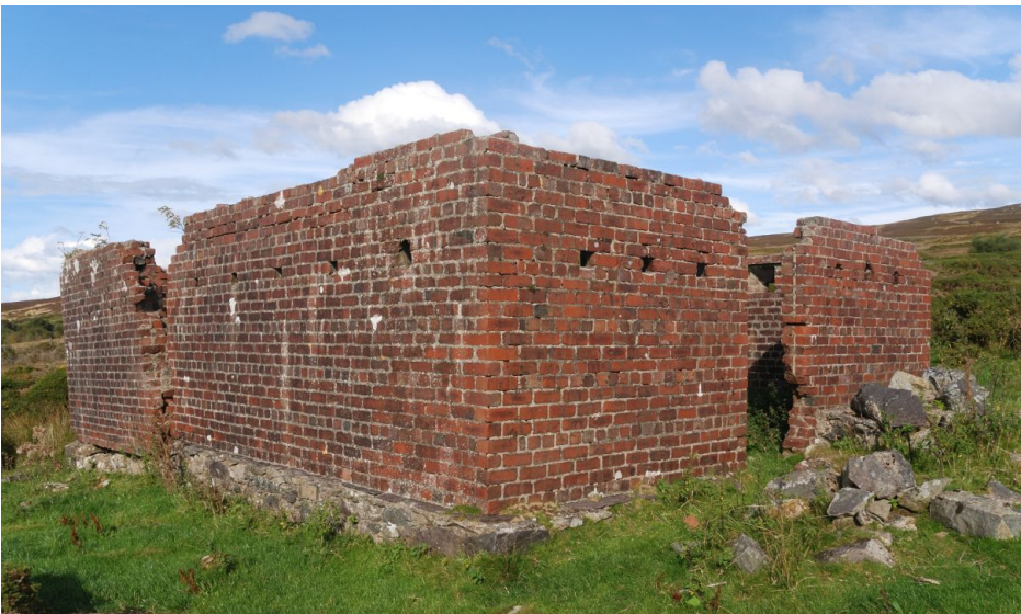
Left: blockhouse 2, southern elevation, with remnant porch, in front of doorway, western elevation to the right.
