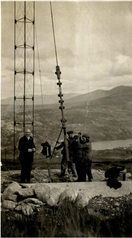
138. Tensioning of one of the stay cables using rods to adjust the large threaded turnbuckles. Probably Mast 15, anchor A. Grounding connections and straps are not installed as yet in this photograph of January, 1924. Bodleian Special Collections MS.Photogr.c.243, photo 715/x.
