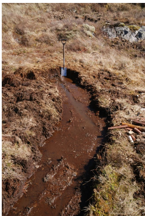
D3 , left: the turn in the double ATI at the north-eastern, 1923 array-facing elevation, evident from the run of the internal drainage channel. The removal of this strip of overlying bog required some six hours' careful removal by small spade.
