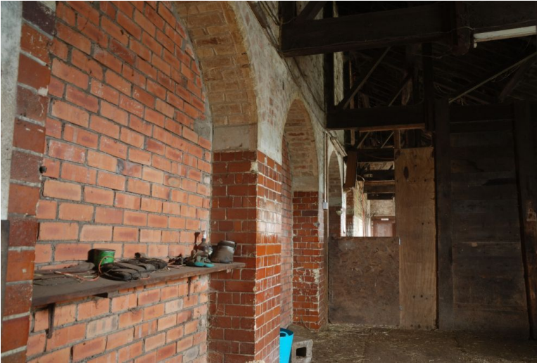
D20 , left: Interior vitreous glazed brick arches at the eastern, antenna-facing side of the transmitter hall. The arch infills are modern and now form part of a horse stable. The roof truss timbers are original and currently in excellent condition, though roof damage now threatens the long-term integrity of the building in general.
