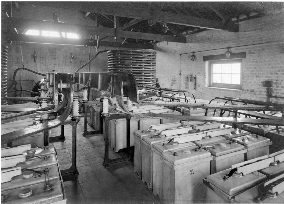
C20. The 'bridging' insulators seen at work, bridging glass-and-oil capacitor tanks of porcelain, in this case, in the transmitter building in 1918. The capacitors were a fundamental part of a resonating, so-called 'tank' circuit, acting in concert with the large inductor coils at background. Strips of copper conductor run inside the insulator channel. Image: Bodleian Special Collections, MS.Photogr.c.243, photograph number P.2072.
