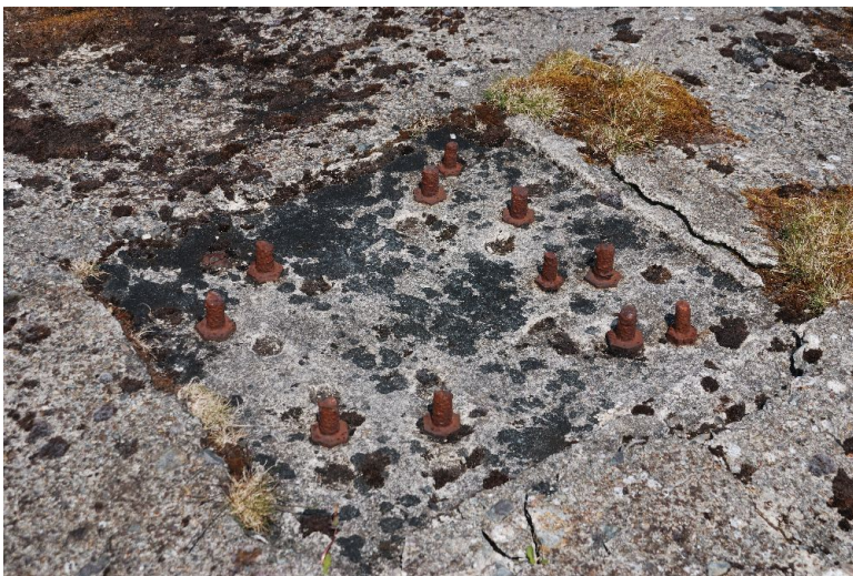
98. Bolts for attaching one of the three feet (Mast 12, foot A) of the 1923 extension masts. Central depression in base 26" x 24". This specific foot has the normal eight securing bolts set into the concrete, but also two, slightly smaller bolts at the inner side. All other pads show impressions of such bolts, which were presumably fixtures on the bottom metalwork of the mast that became fast in what must have been somewhat unset concrete at that point.
