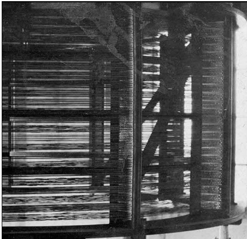
C6. Detail of '9176' insulators seen in their role as inductor wire spacers at the upper inductor house.
