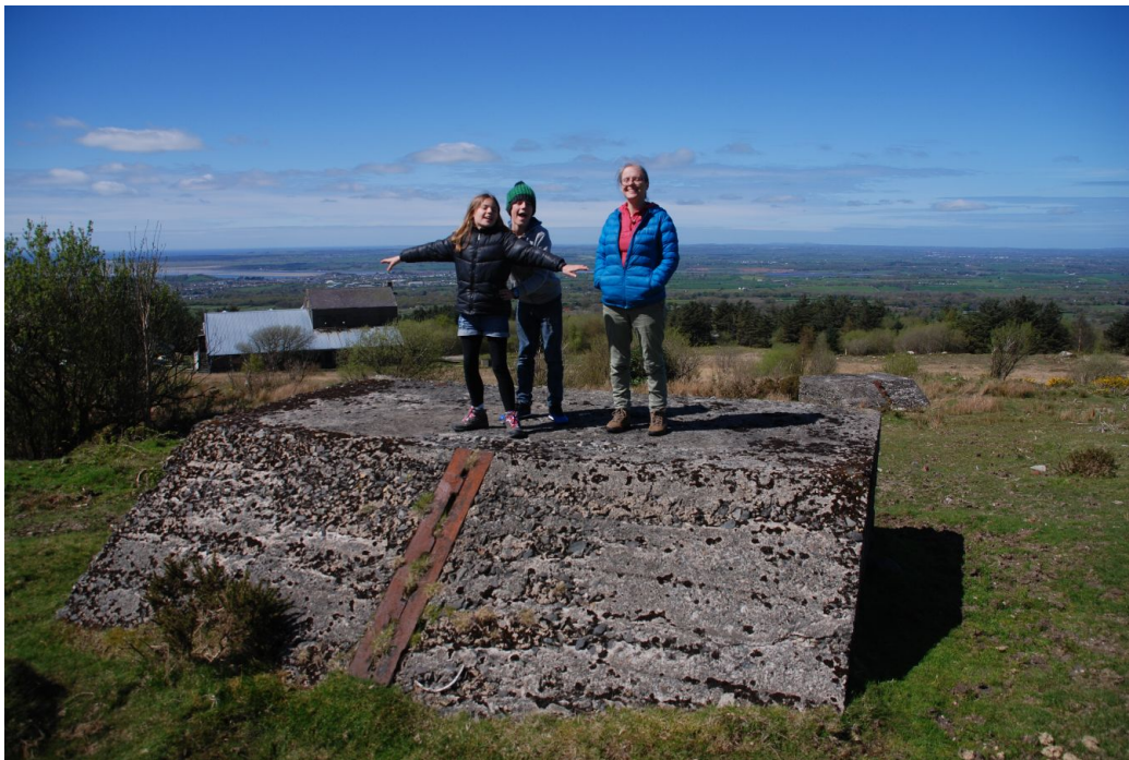
9. A wider, April 2017 view of concrete anchor 3B, with family members for scale! Transmitter buildings seen in background, centre left. The blocks present a 35.5-37 degree (varies slightly between blocks) sloping face, within which stay attachment points are inserted between and bolted to a concreted-in, \frac{1}{4} "-thick, pair of 4"x4" 'L'-section steel retainers, 7' long (slot between is 1.5" wide). Anchors 143" x 124", height variable according to surrounding ground, typically about 45". Anchor fixings 4.25" long. Their mass, some 98 tons ('Trans-Ocean Wireless Telegraphy, New Transatlantic Service, The English [sic] Station Described'; The Wireless World, July 1914, p. 218) has led to at least two of the anchor bases tipping in the peaty ground; 10D by 3 degrees and 4C by 5 degrees. Anchor 4B is in poor condition, but because of this, allows the internal anchor steelwork to be understood (see 123, 124).
