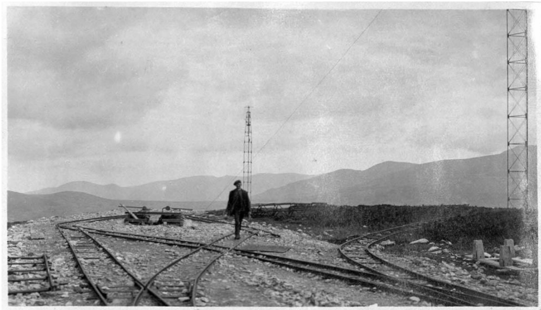
139. The extensive trackway for distribution of construction material, near Cefn Du summit, somewhat to the south of the photograph at 136. The incline down to the majority of the extension site lies directly behind the gentleman, as does the very-nearly completed Mast 15. Mast 14 at extreme right. The incline brake pulleys are seen between the track crossover. The flat saddle in the mountains at centre left is the Mynydd Llandegai and Penrhyn slate quarry area. Bodleian Special Collections MS.Photogr.c.243, photo 710/x dated January 1924.
