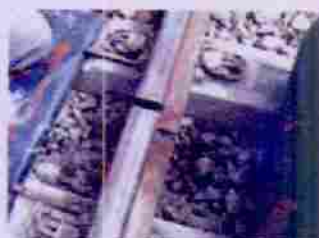
Figure 8.15: Gaps are left in railway tracks to compensate thermal expansion during hot season.
