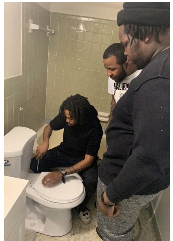
The building maintenance scholars received hands-on certification training to successfully install a toilet.
