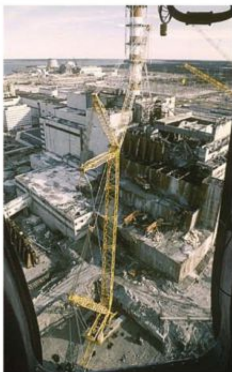
FIGURE 15.2.8 The remains of the Chernobyl nuclear power station in the Ukraine soon after the disaster in 1986.
