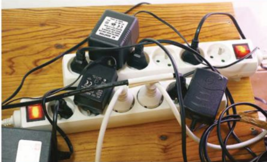
FIGURE 4.3.6 Overuse of power boards and double adaptors can cause overloading of circuits. This can cause wires and components to overheat and start a fire.
