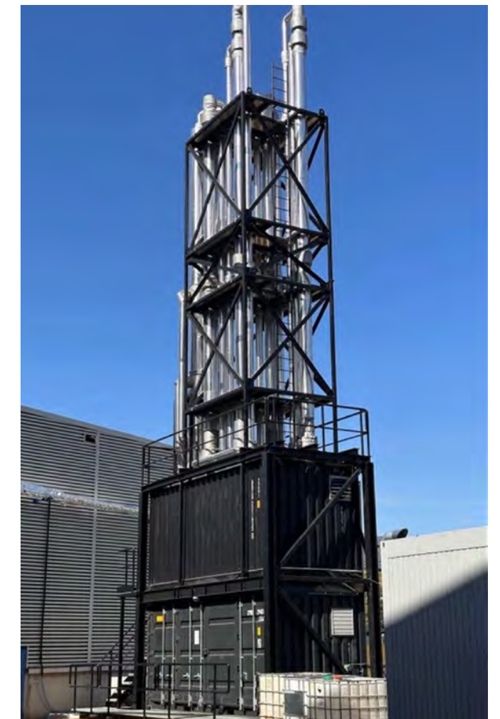
CapsolGo® unit 2 at German EfW (Energy-from-Waste) plant.
