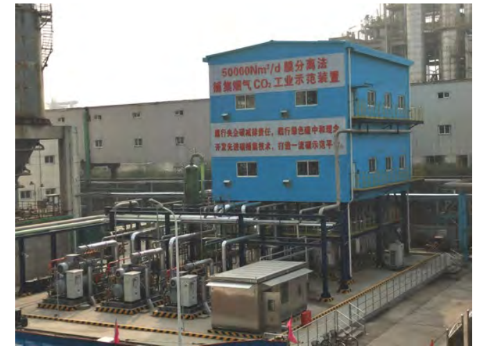
Figure 3: 50000Nm 3 /d membrane separation demonstration
