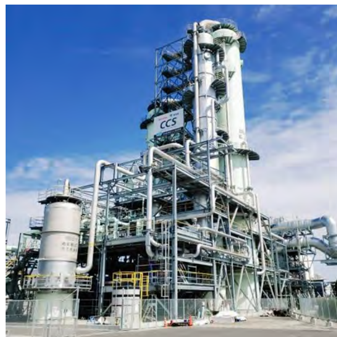
Picture of Demonstration plant of Ministry of the Environment, Japan
