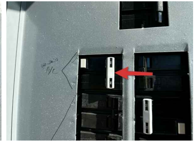
A/C on 50 amp breaker
