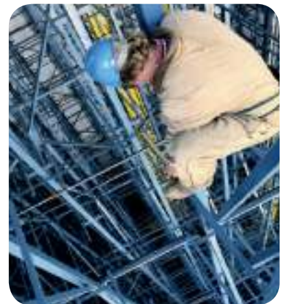
Work at height
