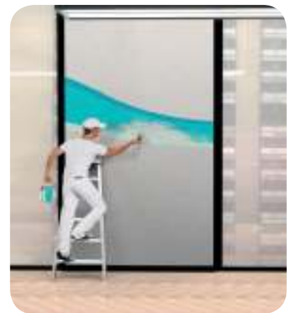
Even minor temporary work presents risk
