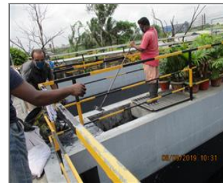
Photo of non-conformity Workers were not using hand gloves in the ETP area.JPG
