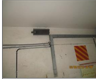
Photo of fire safety equipment PA System.JPG
