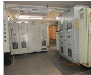
External photo(s) of the production unit(s) Sub-station.JPG
