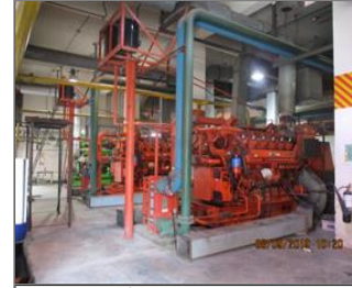
External photo(s) of the production unit(s) Generator.JPG
