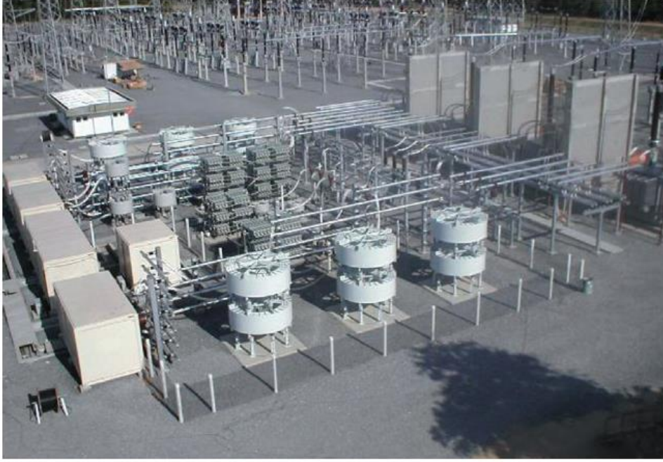
شكل 11-18 : SVC ±250 MVAR in Brazil
