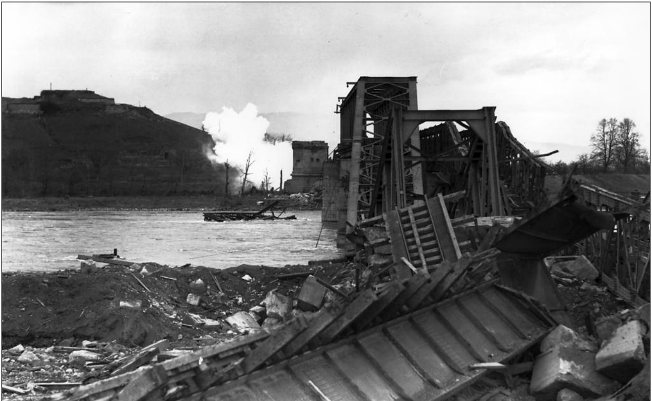
The demolition of the last bridge across the Rhine was the final act in the battle for Alsace (also referred to in the history books as the Battle of the Colmar Pocket), and the 1ère Armée announced that the campaign officially ended at 8 a.m. on February 9. This picture of the wrecked railway bridge at
