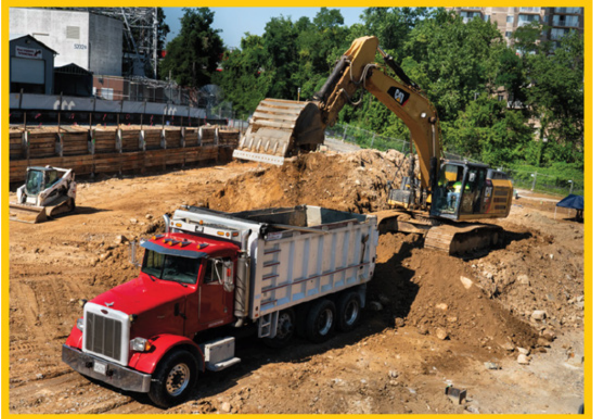
July 27, 2020 approximately 50 dump trucks removed unscreened soil from the cemetery. Photo by Gail Rebhan
