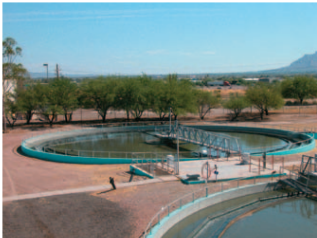
Figure 26.6 Primary treatment of sewage. Here, suspended organic solids settle out as primary sludge. Photo courtesy K. L. Josephson.
