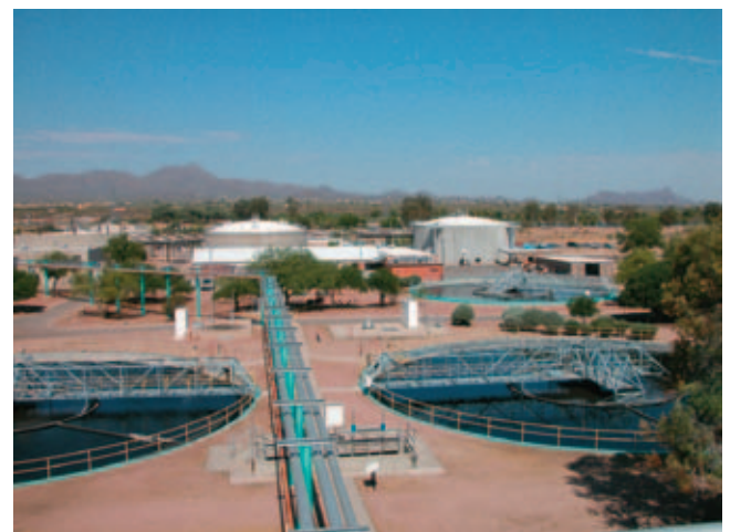
Figure 26.10 Three clarifiers (foreground—blue) and two anaerobic sludge digesters (background—white). Photo courtesy K. L. Josephson.
