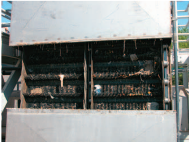
Figure 26.4 Removal of large debris from sewage via a “bar screen.” Photo courtesy K. L. Josephson.
