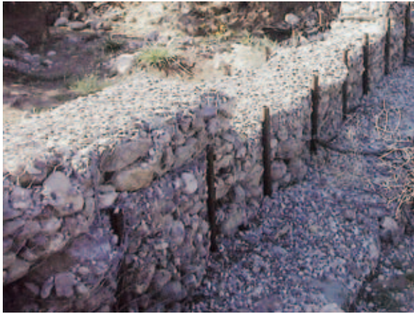
Figure 16.7 A rock-filled dam erosion control structure. From Environmental Monitoring and Characterization © 2004, Elsevier Academic Press, San Diego, CA.
