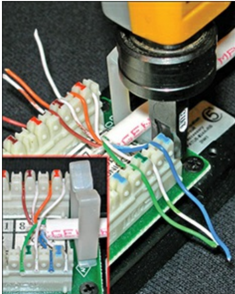
FIGURE 6.18 Punchdown tool inserting wires into an IDC
