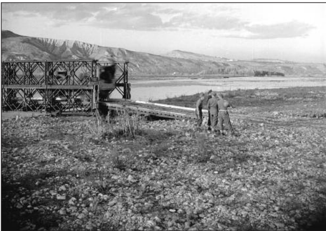
Left: On November 30, New Zealand engineers opened Tiki Bridge, a Class 24 double-double Bailey, adjacent to and downstream from Heartbeat Bridge. This was the first bridge capable of taking tanks. Raised high above the river with bulldozed
