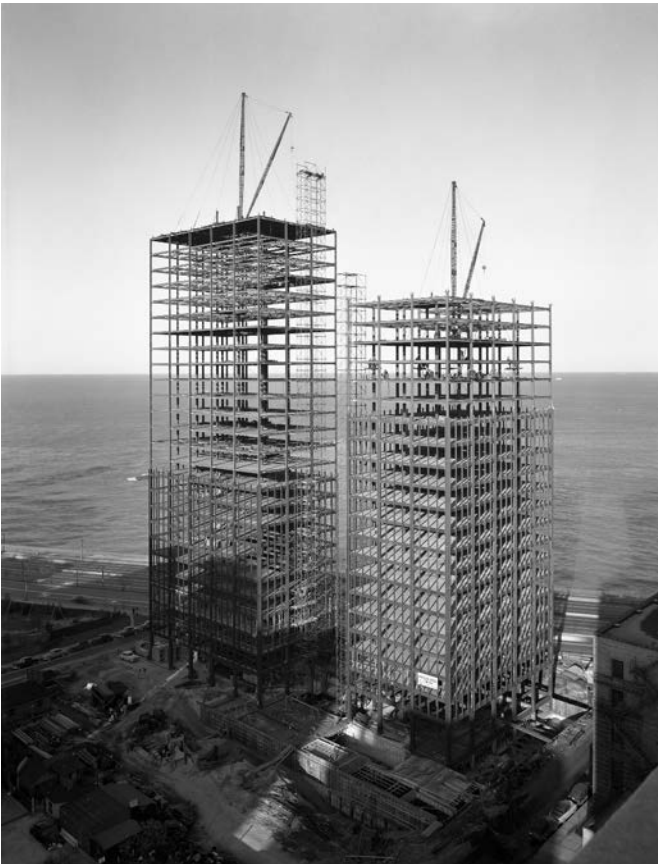
3.20. Steel frame of the Lake Shore Drive Apartment towers under construction, designed by Ludwig Mies van der Rohe, 1948–1951. Photo by Hedrich Blessing. Chicago History Museum, negative HB-1380914.
