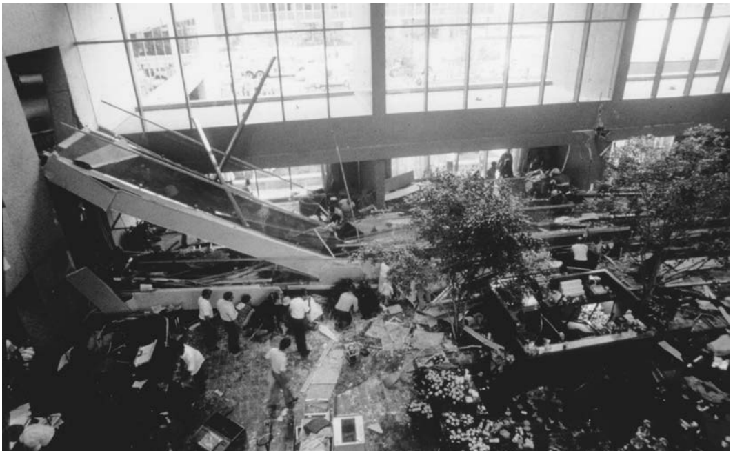
3.49. Hyatt Regency Hotel, Kansas City, Missouri, built 1978–1980; the skybridges collapsed July 17, 1981. Photo: From The Kansas City Star , July 18, 1981 © 1981 McClatchy. All rights reserved. Used by permission and protected by the Copyright Laws of the United States. The printing, copying, redistribution, or retransmission of this Content without express written permission is prohibited.
