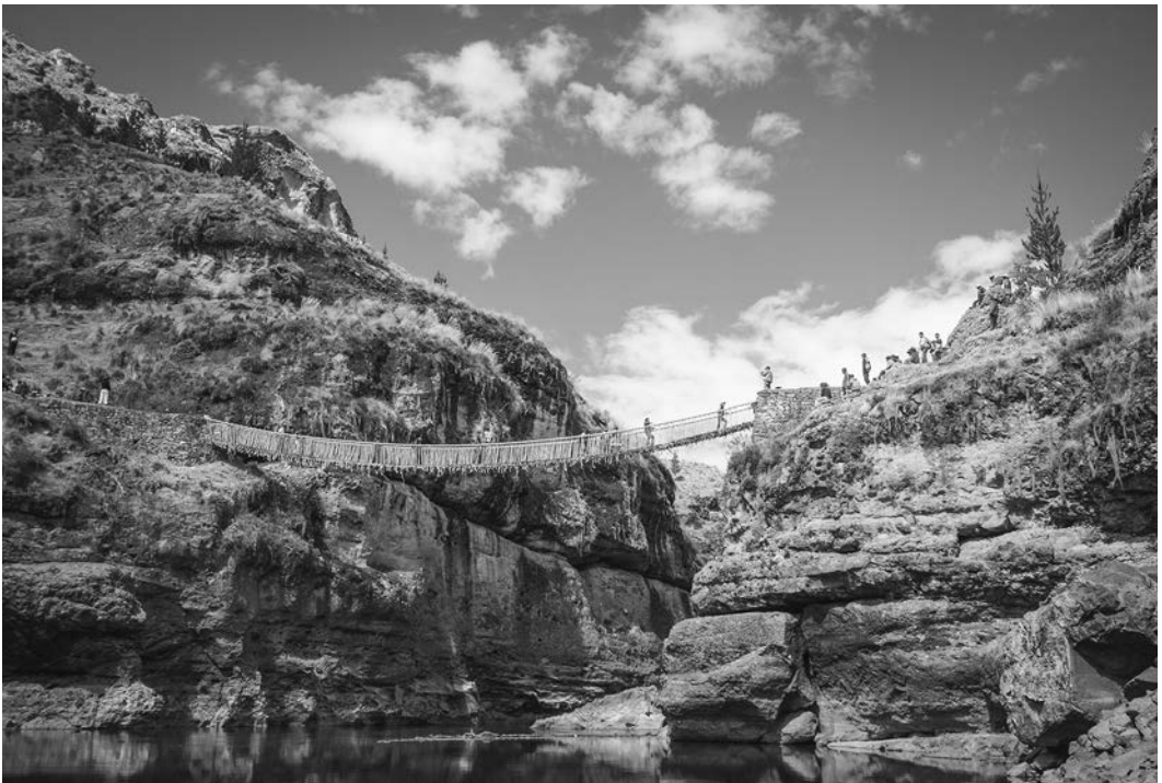
3.40. Qeswachaka suspension bridge, over the Apurimac River, 62 miles from Cuzco, Peru, first built well before 1533. Photo: Isaiah Brookshire.
