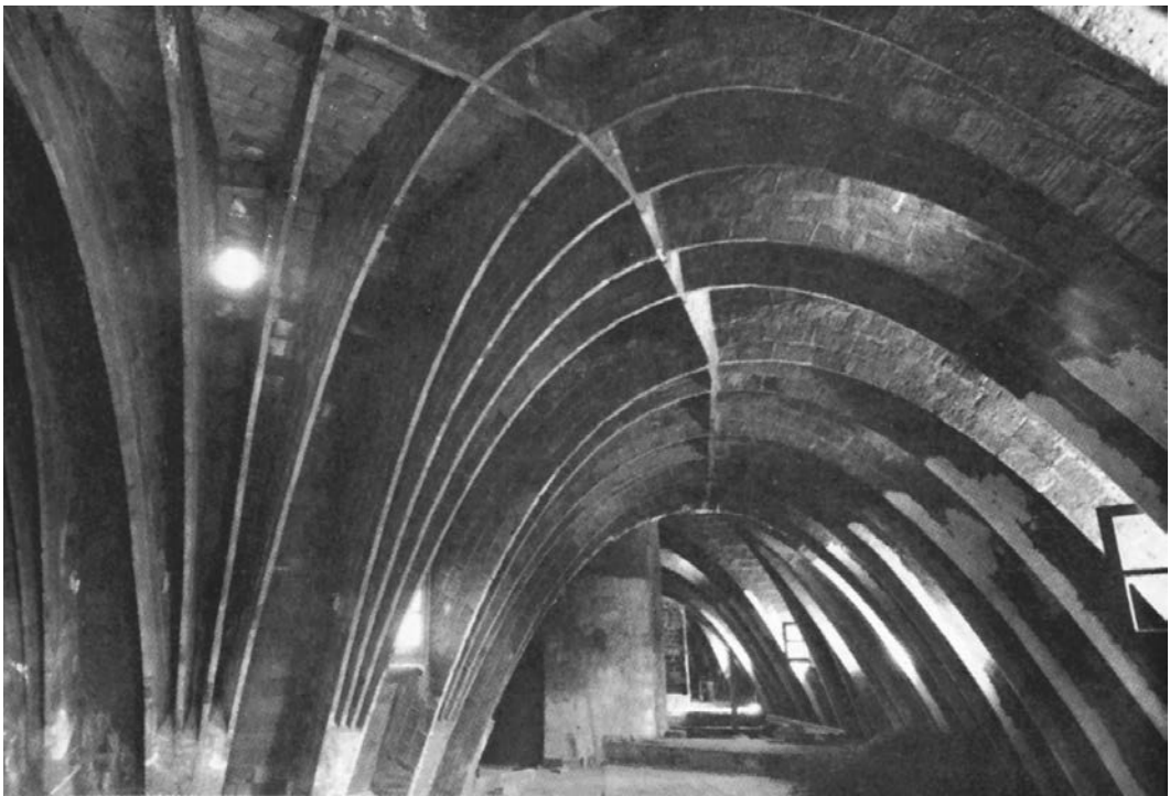
19.3. Casa Milá. The undulating roof of the attic level is formed of arched tile vaults supported by thin parabolic diaphragm arches. Photo: Ampliaciones y Reproducciones MAS, Barcelona.
