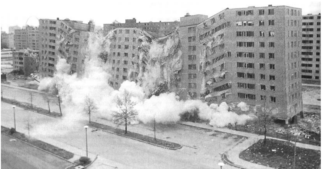
19.56. Dynamiting the Pruitt-Igoe Housing Complex, Saint Louis, Missouri. At 3:32 p.m., July 15, 1972, the first charges of dynamite were detonated, demolishing what had once been considered a model public housing complex. All the vaunted high ideals of International Modern architecture seemed to come crashing down with it. Photo: St. Louis Post-Dispatch.
