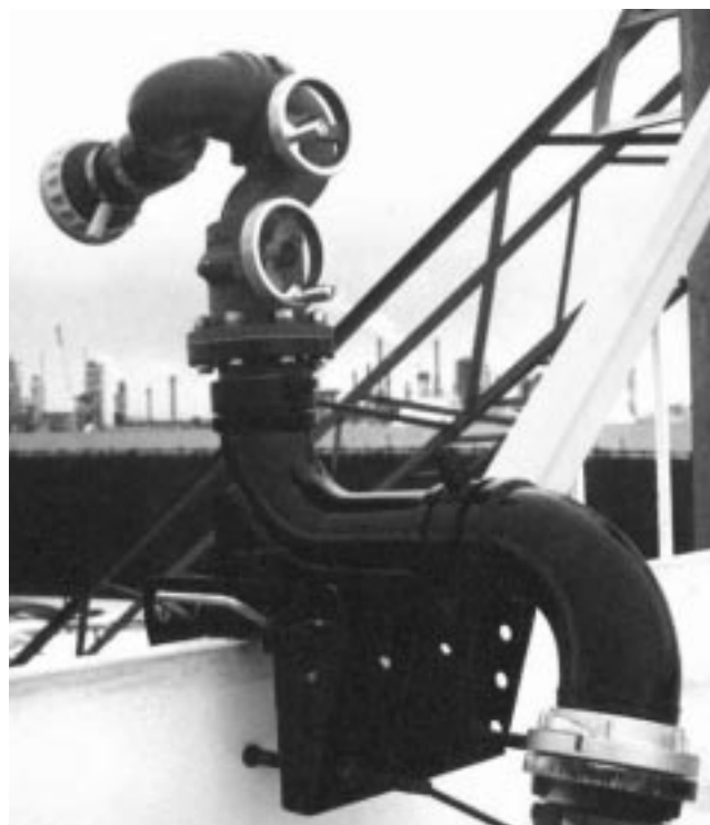
Figure 14—Special Portable Monitor Attached to Edge of Floating Tank Roof to Fight Rim Seal Fires
