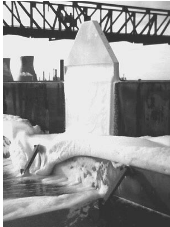
Figure 12—Foam for Seals Flowing into Foam Dam from Permanently Installed Foam Chamber
