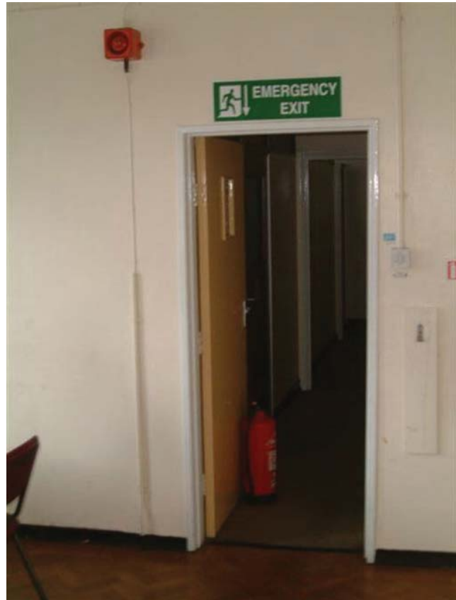
Figure 4.16 Routine violations of basic safety systems indicate a poor safety culture – wedged fire door
