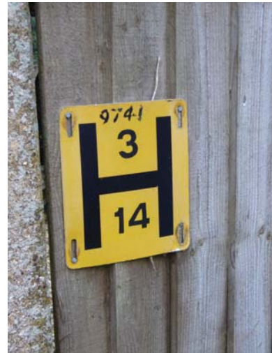
Figure 9.89 Fire hydrant indicator plate
