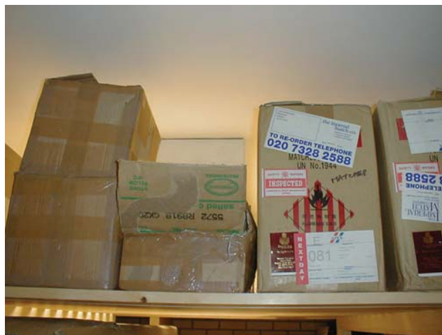
Figure 7.16 Boxes containing matches being stored adjacent to a light fitting
