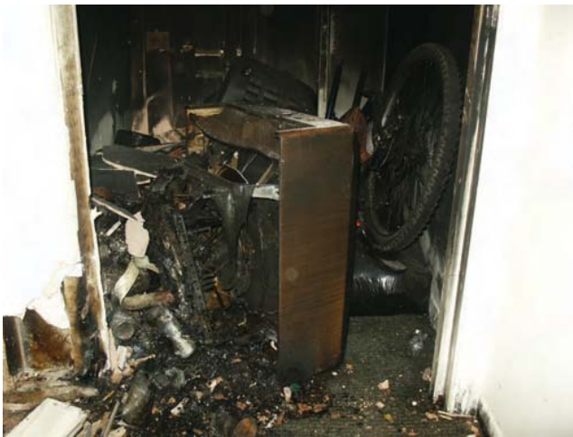
Figure 12.9 Damage to records and stored items following an arson attack
