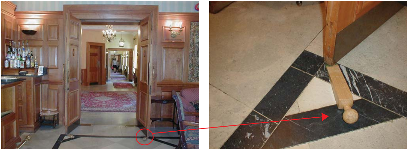
Figure 9.39 Example of abuse of fire compartmentation by the use of door wedges
