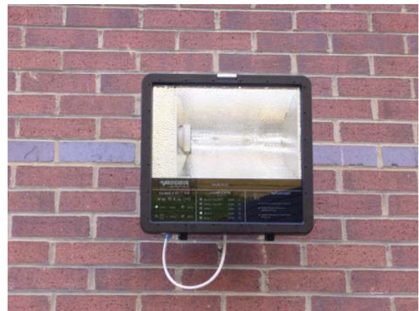
Figure 8.9 Typical security lighting
