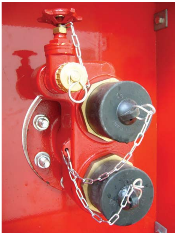
Figure 9.88 Dry riser outlet
