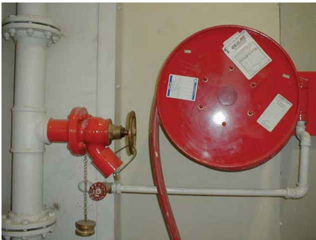
Figure 3.3 Fire fighting equipment must be appropriate and adequately maintained
