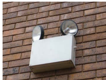
Figure 9.51 Emergency lighting unit
