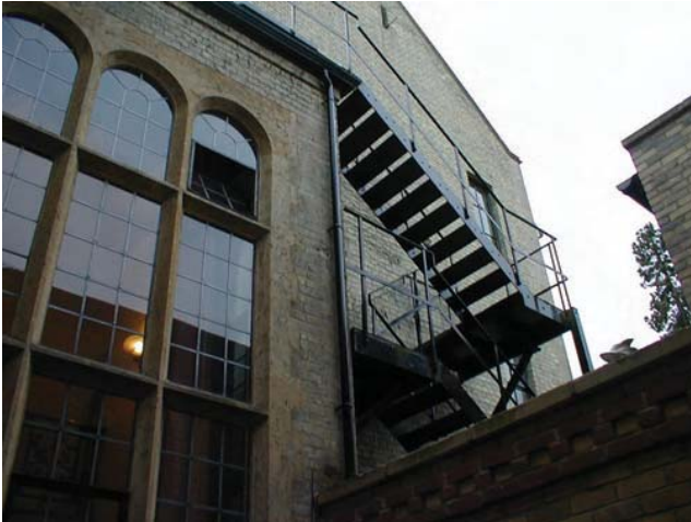
Figure 9.46 Metal fire escape above non-FR glazing – note open window
