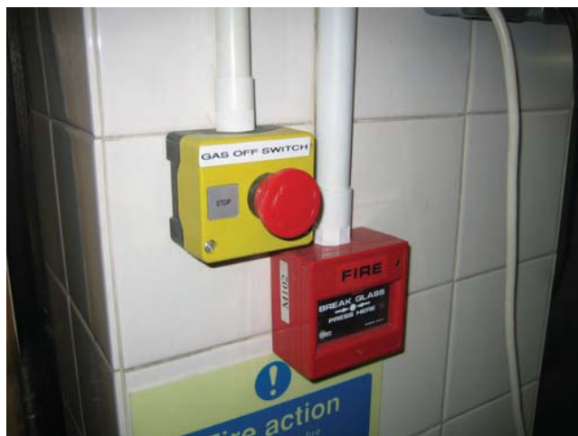
Figure 3.10 Isolation switch for gas-fired kitchen equipment
