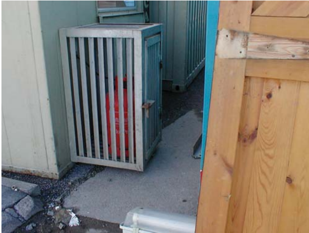
Figure 8.20 LPG cylinder storage facility
