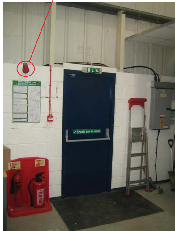
Figure 9.82 An example of a combined audible and visual fire alarm installed in a potentially noisy workplace
