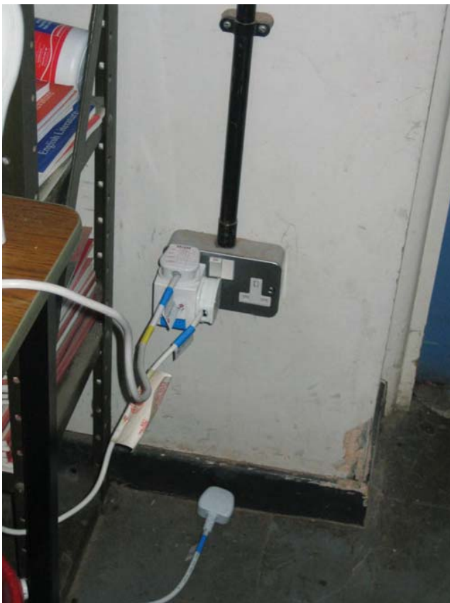
Figure 11.6 Misuse of electrical adaptors
