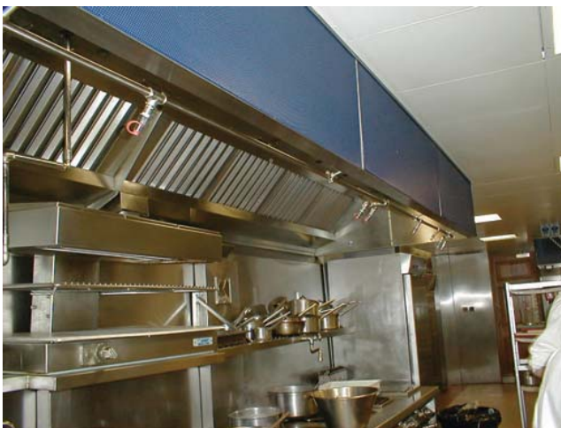
Figure 8.14 Gas cooking installation showing fixed fire fighting equipment
