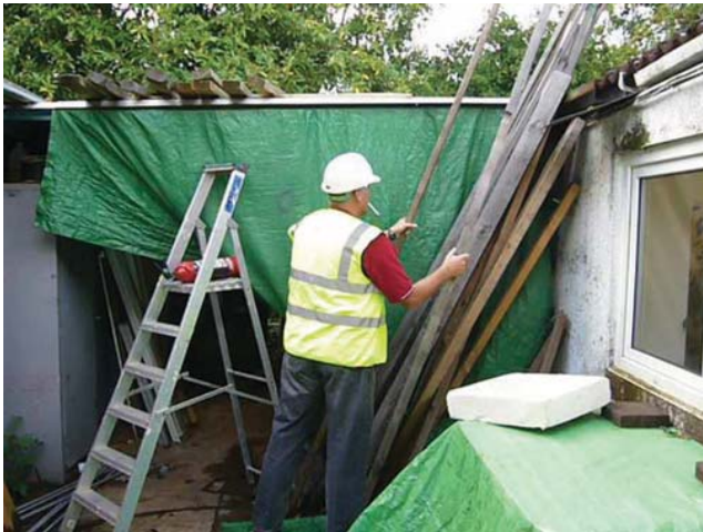
Figure 5.9 Building contractors have the potential to increase fire risk
