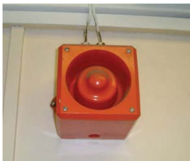
Figure 9.81 Audible fire alarm
