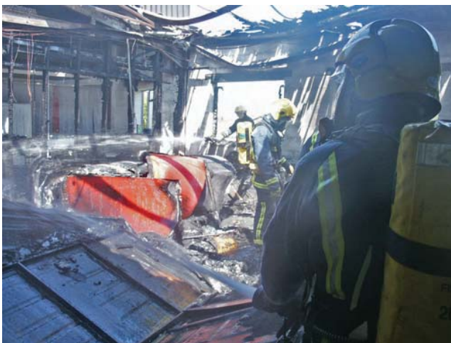
Figure 1.1 Aftermath of fire – the cost of failing to manage fire safety
