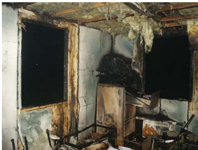
Figure 12.1 The consequences of failing to monitor events can lead to serious accidents
