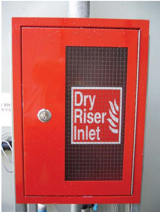
Figure 9.87 Dry riser inlet
