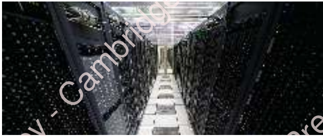
Figure 13.15: Data storage facility.
