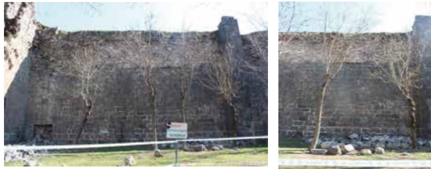
Fig. 28 and 29: Wall between the 19th and 18th Towers: New dense stones have fallen from the surface. Spills, in particular, cover a large area in the upper part of the wall between the buttress and the 18th tower. The inner filling of the small secondary door in the wall has also collapsed.
