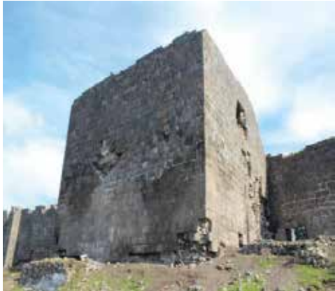
Fig. 12: 29th Tower: There is damage to the surface texture caused by new stone spills, and the risk of stone falling continues.
