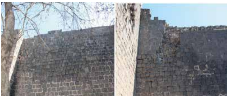
Fig. 17, 18: Wall between 24th and 23rd Tower: The joint filler has collapsed. In addition, new stone falls have occurred in the section of the wall where the surface stones were previously poured. The risk of further surface stone spillage remains in this area.
