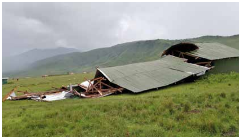
Fig. 3: A house in Oloirobi destroyed by the authorities. Its owner is not allowed to repair it. Photo: Marko Kipuyo
