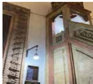
Fig. 73: It was observed that there is a vertical crack descending from top to bottom at the junction of the minber with the eastern wall.
