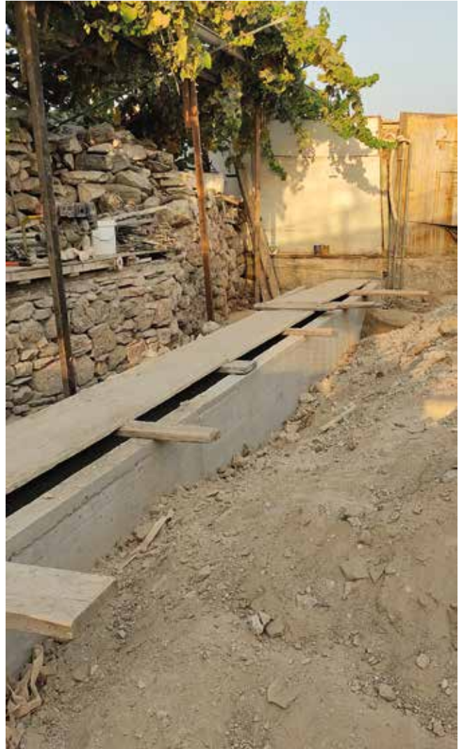
Fig. 16: The same area depicted in Fig. 15, as it was in summer 2021, looking south-west. On the south side, the reinforced concrete channel that was later covered with the metal mesh seen in Fig. 15. The area is not yet filled and paved with reinforced concrete as in Fig. 15 and 17.
