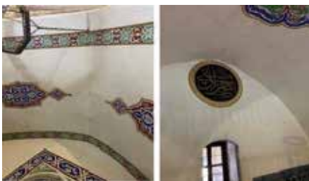
Fig. 70, 71: There are cracks on the vault keystone down to the stained glass windows on the eastern part of the entrance hall, the prayer hall ( harim ), and the prayer hall for women ( kadınlar mahfili ) located on the western part of the mosque. Again, there is a crack starting from the vault and extending to the window above the entrance and in the muezzin's mahfil . It should be analysed whether this is a plaster or a structural crack.
