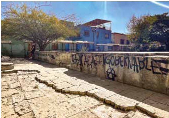
Fig. 5: Damages to Plazuela del Carmen Alto.
