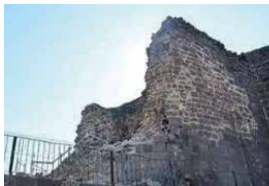
Fig. 52: 75th Tower: Falls from the inner filling and surface stones on the eastern façade were caused by the earthquake.
