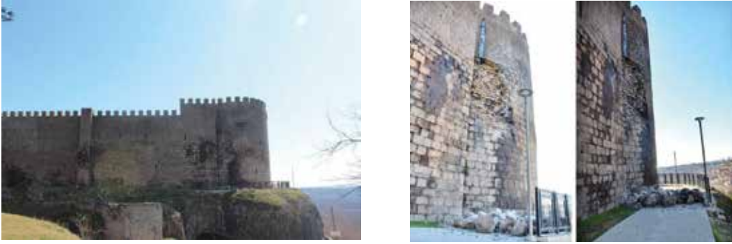
Fig. 2–4: 52th Keçi Tower, 09.02.202: It was observed that the surface stones were poured on the western face of the tower, and vertical cracks were formed on the wall infill in the pouring area. Furthermore, the water flowing from the gargoyles flowed onto the wall surface, causing the binding mortar to soften and losing its binding properties. In addition, it was noted that the expansion and contraction caused by the freezing and thawing of the water flowing due to the temperature difference between day and night in the winter also created a negative effect and pose a risk.
