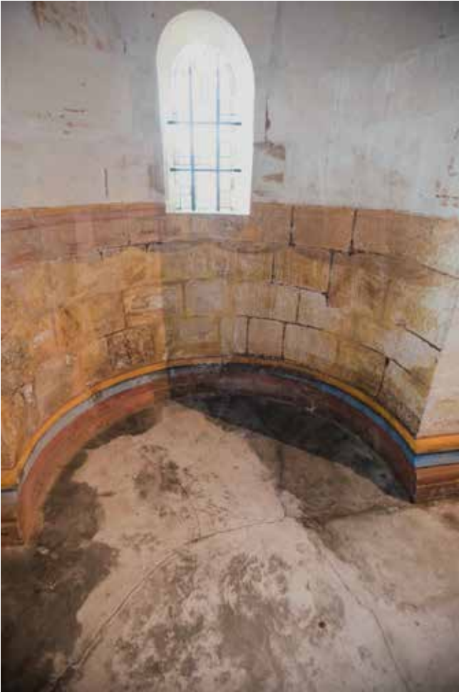
Fig. 6: Moisture and cracks in the floor of St. Ulrich's Chapel. Photo: Henning Frase
