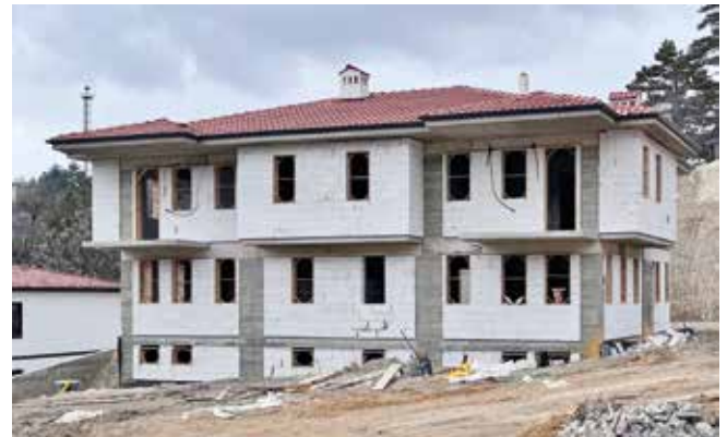
Fig. 2: Reinforced concrete house under construction in Safranbolu Çukur. The weakness of the design becomes evident in the absence of window lintels on the upper floor. The geomorphology of the place was destroyed by making very deep trenches.
