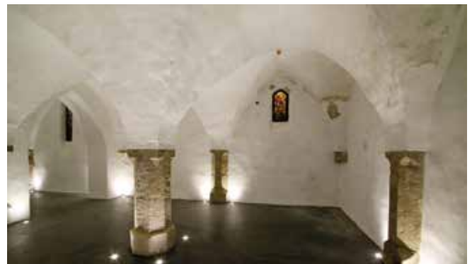
Fig. 3: Damage caused by moisture penetration in the cellar vault of the town hall.
