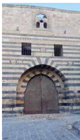
Fig. 38: Khan al-Wazir: Bulging at the top of the façade and some of its parts falling off
