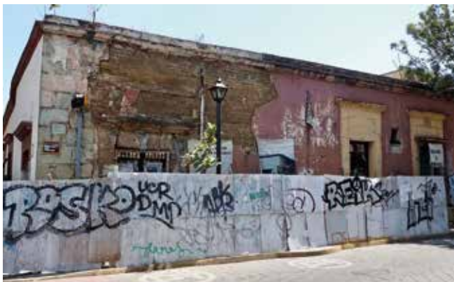
Fig. 2: Buildings' deterioration and vandalism in the historical centre.
