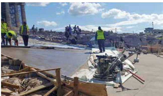
Fig. 2: The area in front of the east front of the Propylaea, in the process of being paved with reinforced concrete, covering over the face of the living rock. The wet cement on the picture's left end is covering the plastic sheet and metal mesh in Figure 1. View from the northeast corner of the platform. Above left, the west end of the Parthenon.
