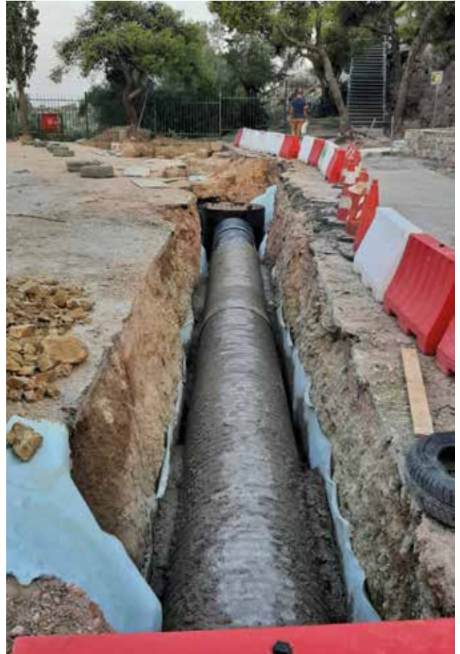
Fig. 20: A view of the ditch surrounded by the plastic white and red plastic parapets illustrated in Fig. 19, looking west. The big pipe is being encased in cement that will bear the fill to reach the surrounding ground level (2023). Photo: Tasos Tanoula
