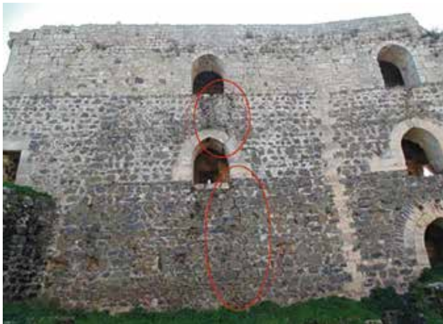
Fig. 1: Collapse of a part of the wall filling, with a height of 5m and width of 1.5m. The filling consists of limestone and basalt and traditional binding components.
