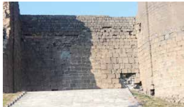
Fig. 58: Wall between 59th and 58th Towers: There are stones fell from the previously masonry-closed gate on the wall.
