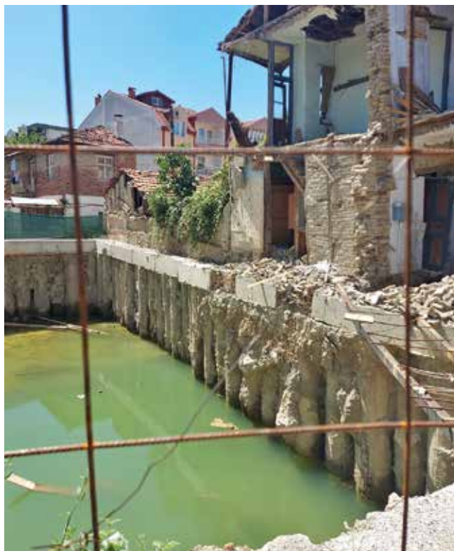
Fig. 3: In the Old Town Core of Ohrid in August 2022, a new construction moves forward with permission. Its height will exceed maxima set in the current Ohrid Region Management Plan.
