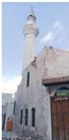
Fig. 37: Ottoman mosque: collapse of newly restored parts.
