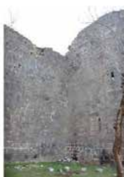
Fig. 26, 27: 19th Tower: New stone falls were noted on the northwest façade's upper corner. Cracks have formed, and the danger remains. There are also new stone falls at the tower's junction with the wall to the north.
