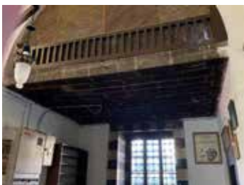
Fig. 72: The stone floor of the eastern mahfil was cracked and the floor sloped slightly towards the bottom. The destruction can be monitored from beneath the floor.
