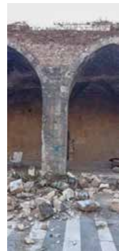
Fig. 39: Partial collapse in many cases
