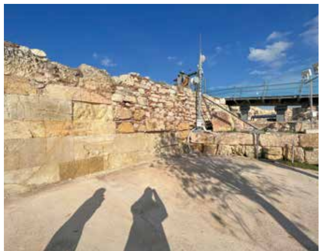
Fig. 17: The same area as in Fig. 15 and 16, looking northeast. The reinforced concrete pavement spreads out to the fifth century B.C. ashlar poros masonry, sealing the lower part of the wall and the access to the antiquities and the living rock underneath.
