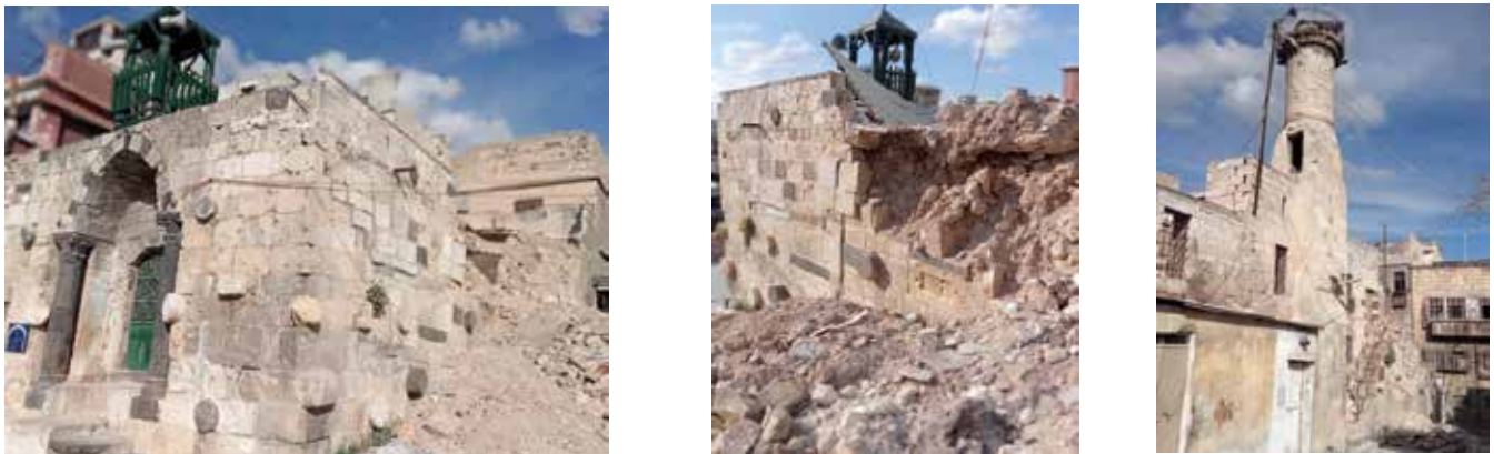
Fig. 5–7: A major collapse in Al-Qiqan Mosque
