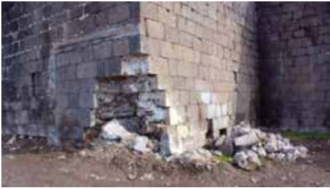
Fig. 11: 30th tower. The tower has new stone falls in its corner.
