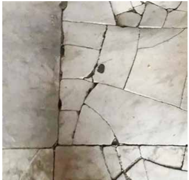
Fig. 5: Damaged marble floor
