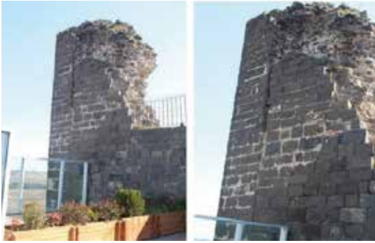
Fig. 53, 54: Corner wall where the North and East Walls meet: Vertical separations on the wall pose a danger.
