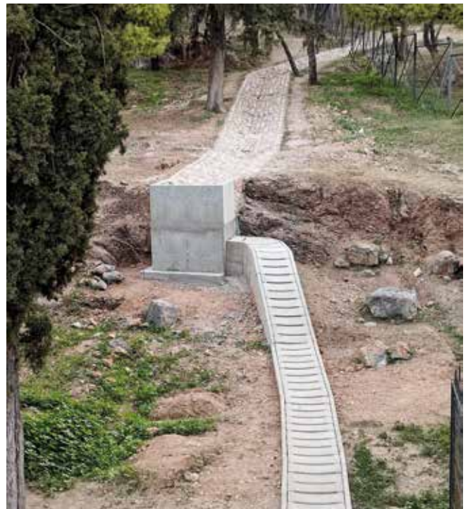
Fig. 22: Another stretch of the drainage system on the slope to the north-west of the Areopagus. Similar structures are made of reinforced concrete and spread out in most of the archaeological site around the Acropolis and the Areopagus (2022). Photo: Tasos Tanoula
