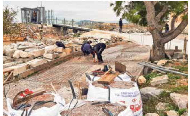
Fig. 12: A pathway out of the boundaries of the tourist's routes on the Acropolis in the process of being paved with reinforced concrete. Above left, the new elevator. Above right, behind the tree the Erechtheion. Photo: Tasos Tanoulas
