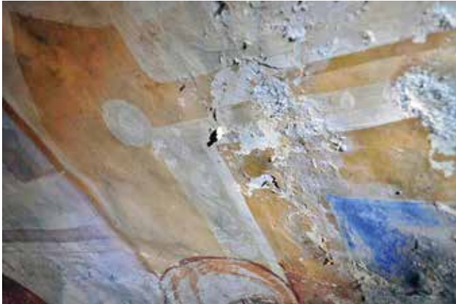
Fig. 4: Painting condition, Northern arm, January 2023. Photo: Chubinashvili Centre
