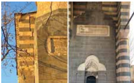
Fig. 68, 69: Behram Paşa Mosque: There is a decomposition at the joint of the last congregation place and the minaret which is found on the north-western corner of the mosque. Similar decomposition is observed on the north and south facades.
