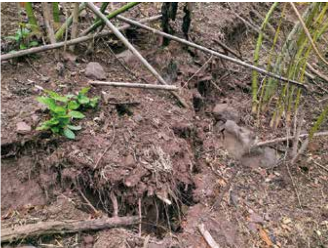
Fig. 7: A crack in this bamboo-covered steep slope hints at an impending landslide.
