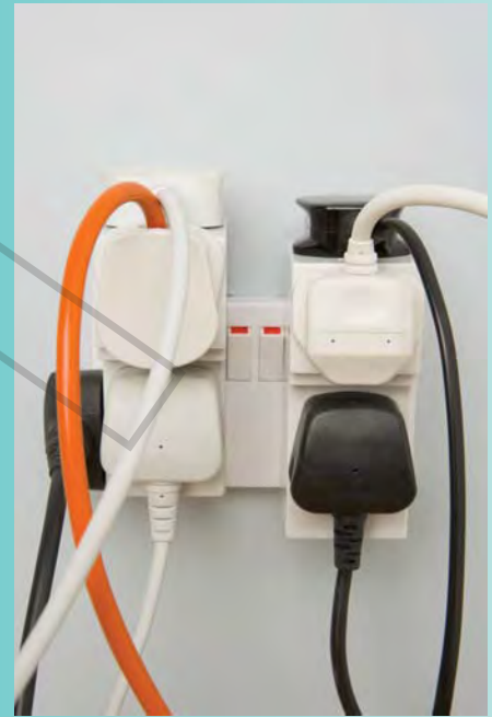
▲ Figure 4.33 An overloaded socket increases the risk of a fire.
