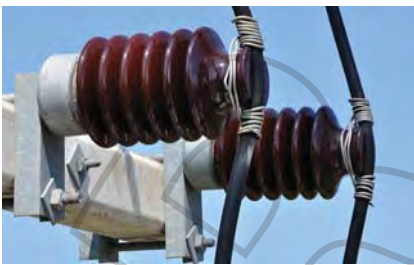
▲ Figure 2.11 These ceramic discs have a very high resistance so that the power line is insulated from the metal pylon.
