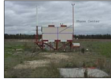
MLS Azimuth guidance station with rectangular azimuth scanning antenna and DME antenna at left Fig 23.2 – F (USGS Photo)
